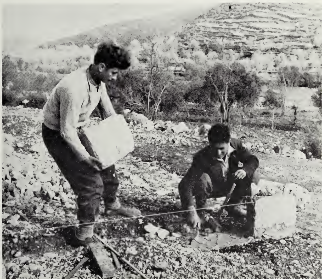
Boys at rural center, Lebanon, learn masonry as they lay foundation for a new poultry house
